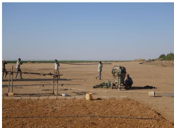
Figure 2. Chinese and Sudanese workers constructing a new ginning factory. Photo by the Author.
